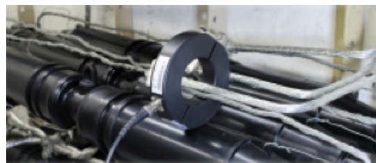
CLAMPS FOR PARTIAL DISCHARGES GROUNDED
