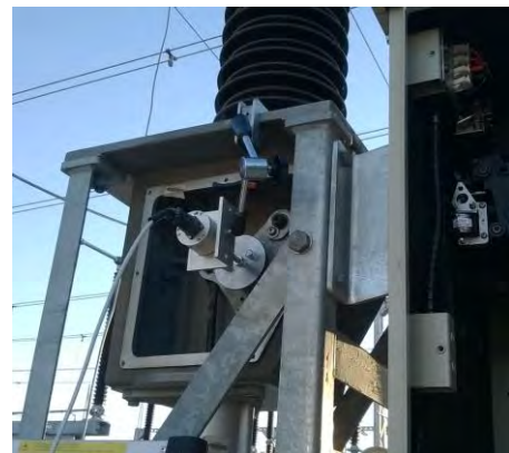
Digital rotary transducer mounted on ABB LTB 245 kV SF6 circuit breaker
