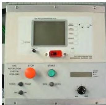
Detail of control panel
